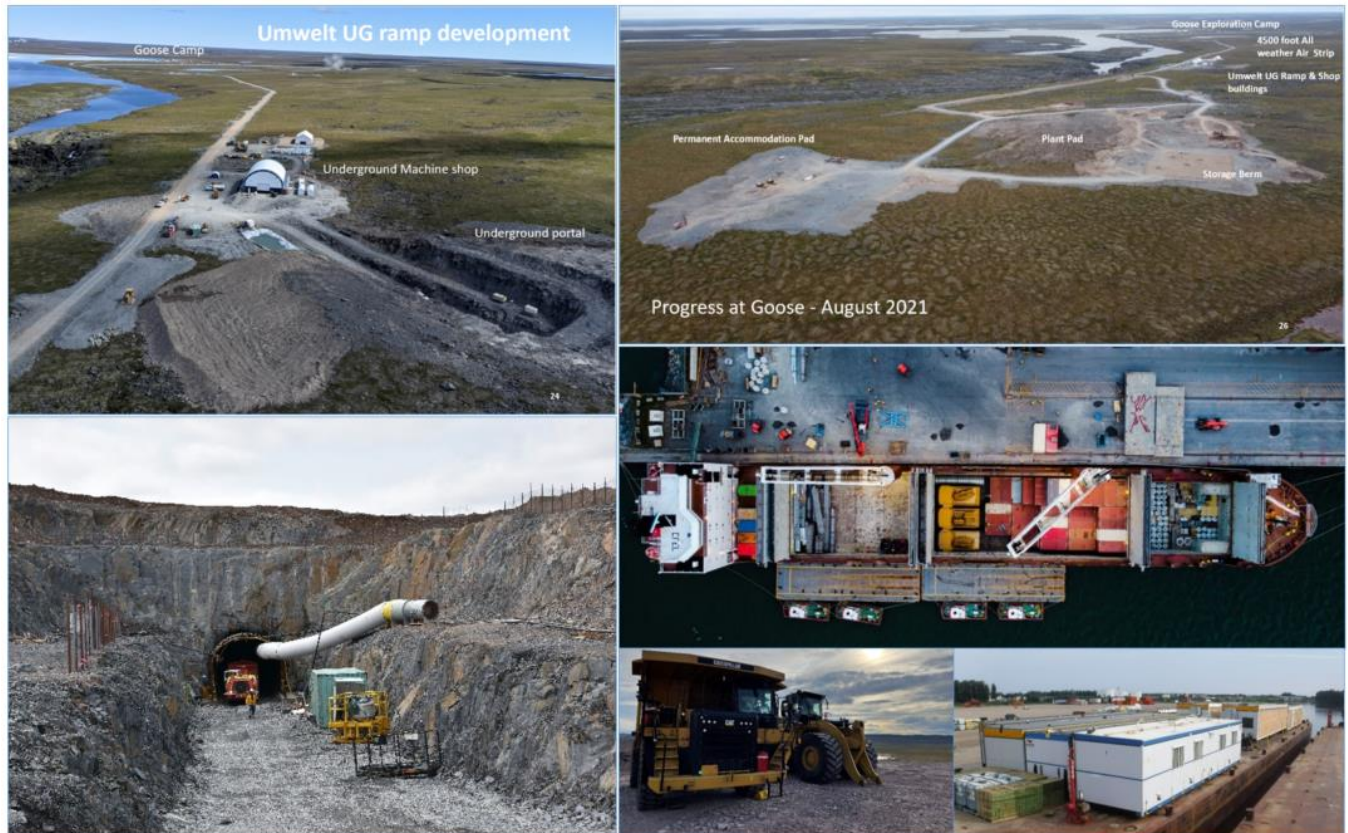
Figure 1. Recent photos of Umwelt UG ramp development, Goose progress overview and sealift
